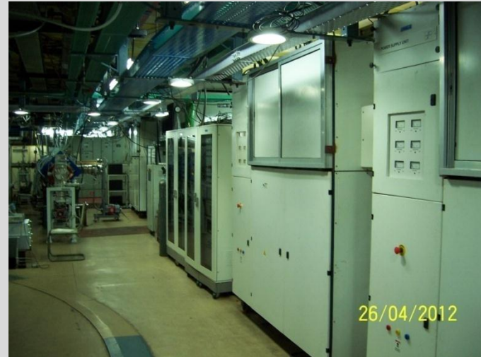
SAMEER Mumbai – RF transmitters
