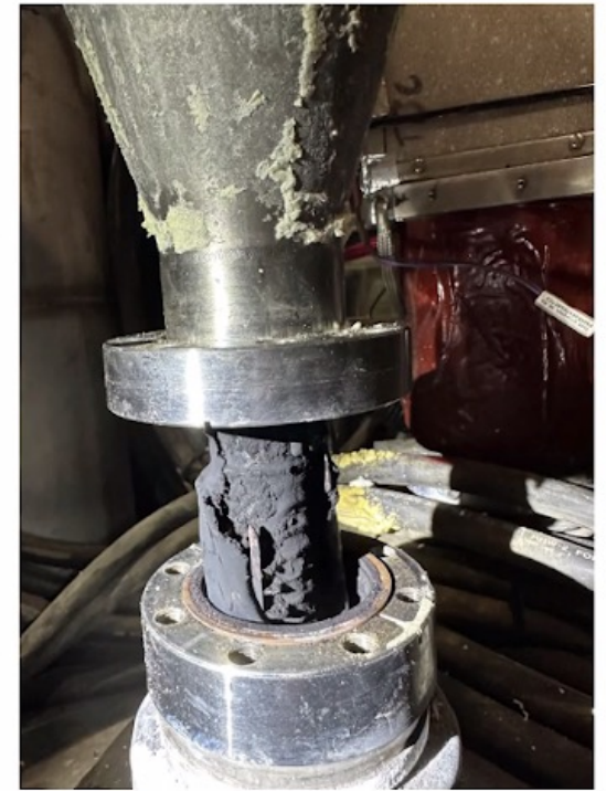
Charred 150 amp feedthrough
