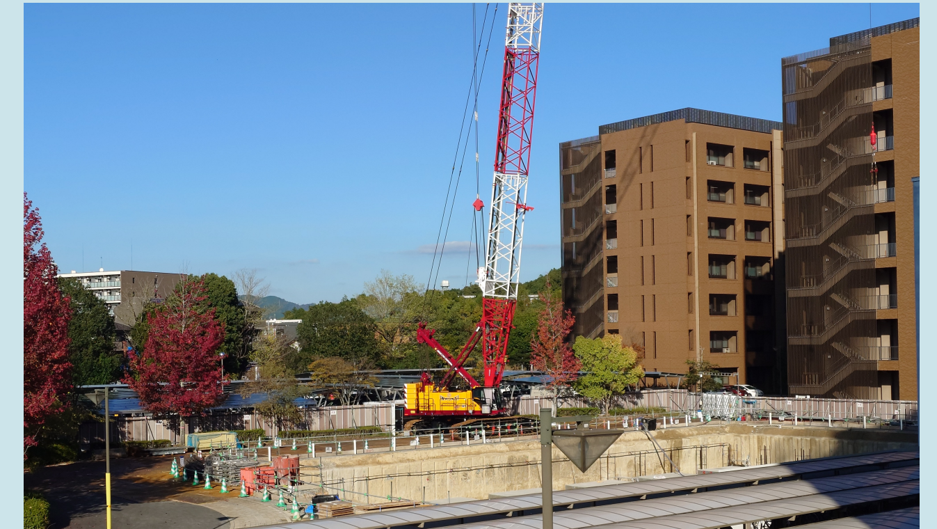
Japan to Join Electron-Ion Collider Accelerator Construction Project; Potential Boost for Quantum Computer Technology
